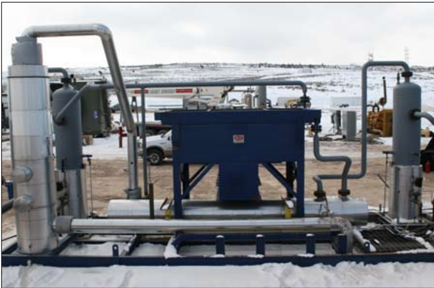
Figure 5 2500 Mscfd X-O 2 oxygen removal unit
