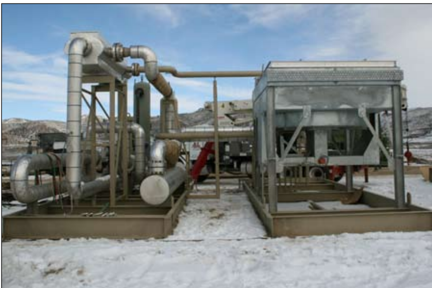
Figure 6 10 000 Mscfd X-O 2 oxygen removal unit
